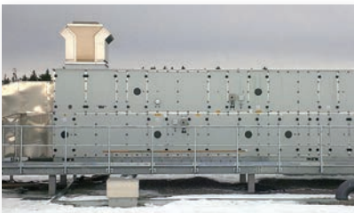
A) Fully assembled rooftop unit
